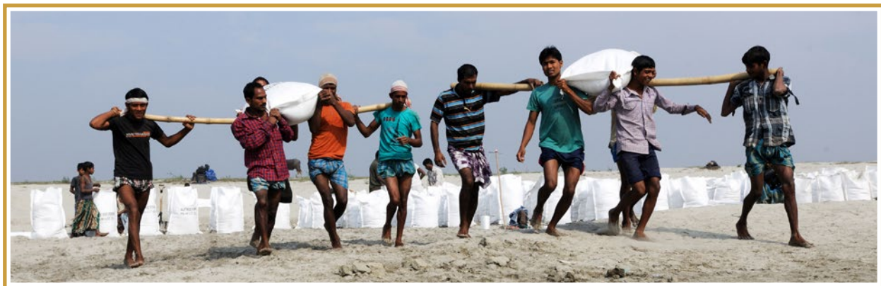
Workers carrying sand filled geo bags to be pitched on the banks of the river Brahmaputra in Gumi village, Guwahati as part of the Assam Integrated Flood and Riverbank Erosion Risk Management Investment Program. Photo: Rakesh Sahai for ADB
